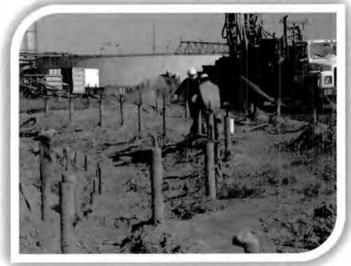
Figure 3.4.1 Uncovered freeze pipes disconnected from supply/return headers
