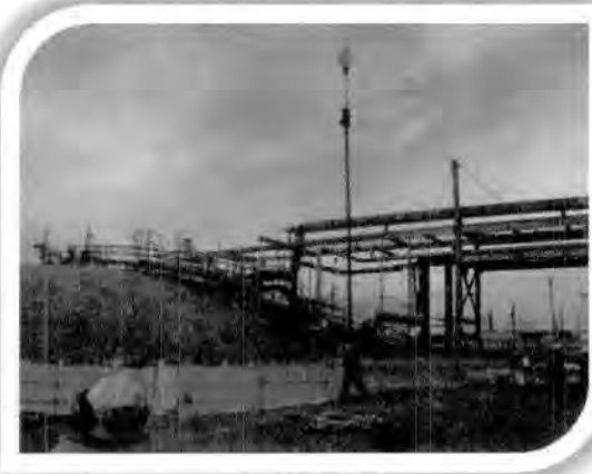
Figure 3.2.2 Removal of pump to shaft to be able to install nitrogen hose
